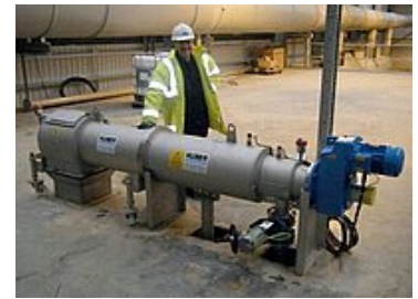
STRAINPRESS® installation on mezzanine floor
