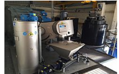
HUBER Disc Thickener S-DISC skid mounted installation at Great Dunmow
