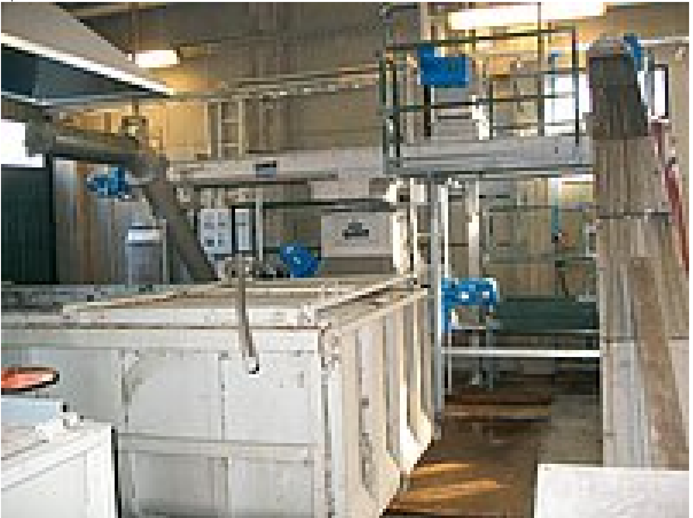
Ro 8T screw conveyors move all screenings to the WAP/SL; visible is the top of its launder tank, the impeller motor and the rising pressure pipe; a highly compressed screenings plug is pushed out of its end
