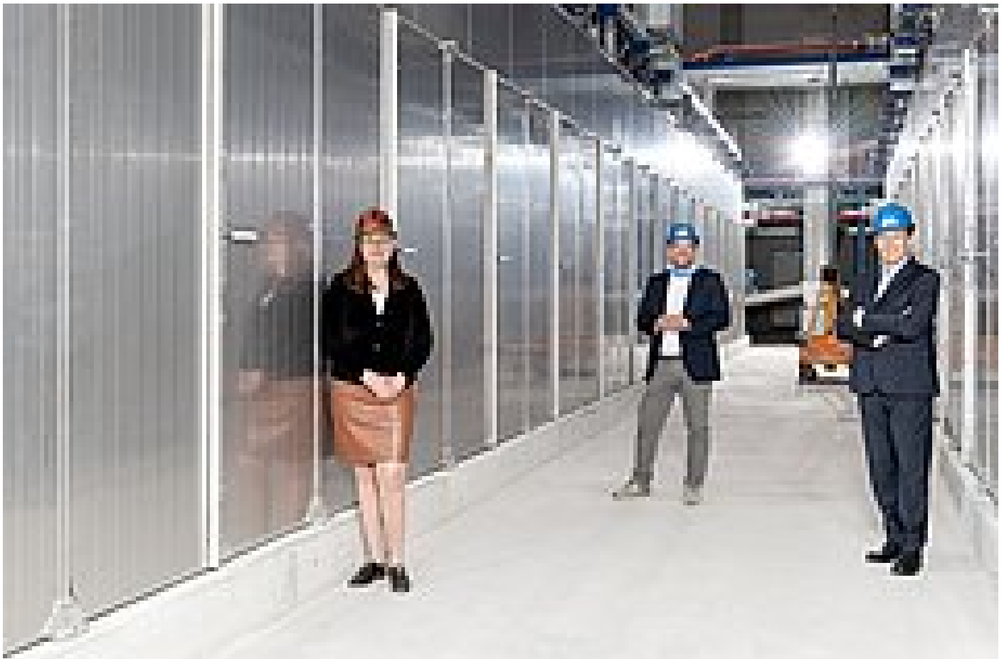
Official start of commissioning on 23 April 2020 by the management and the Lord Mayor began during a press meeting on site [(C) Andreas Berthel]
