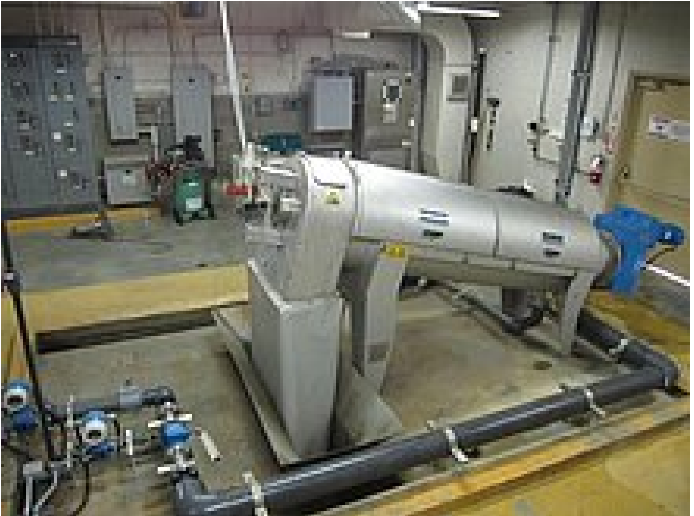
HUBER's Screw Press Q-PRESS® at Cardston's Wastewater Treatment Plant
