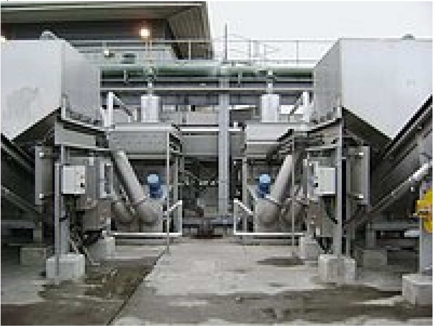
Laundry tanks and rising compaction pipes of the seven WAP/SL units
