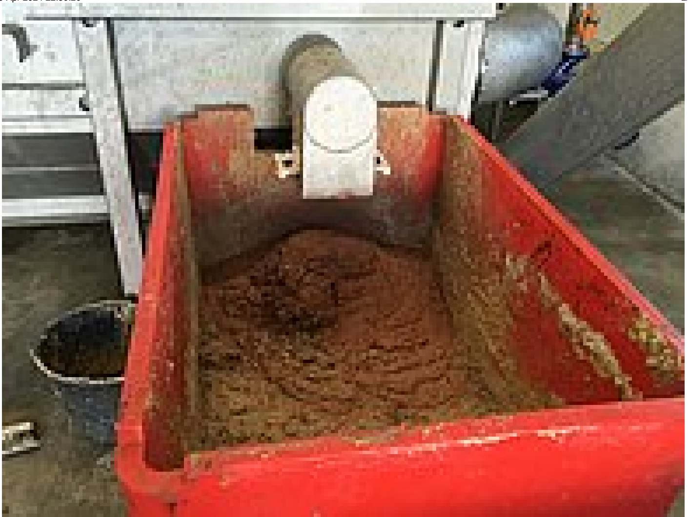
Discharge from the fat separation
