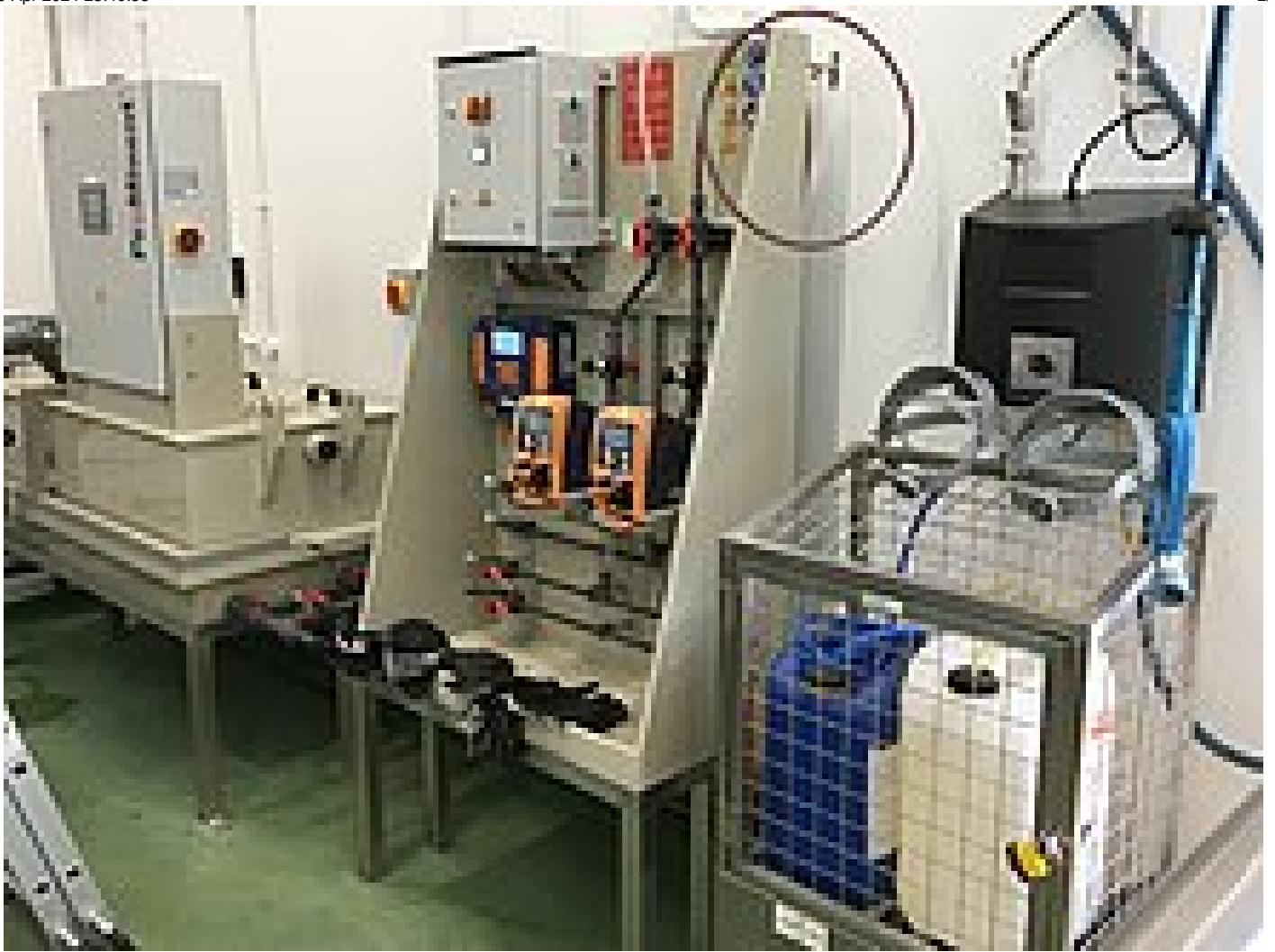
New chemical dosing plant
