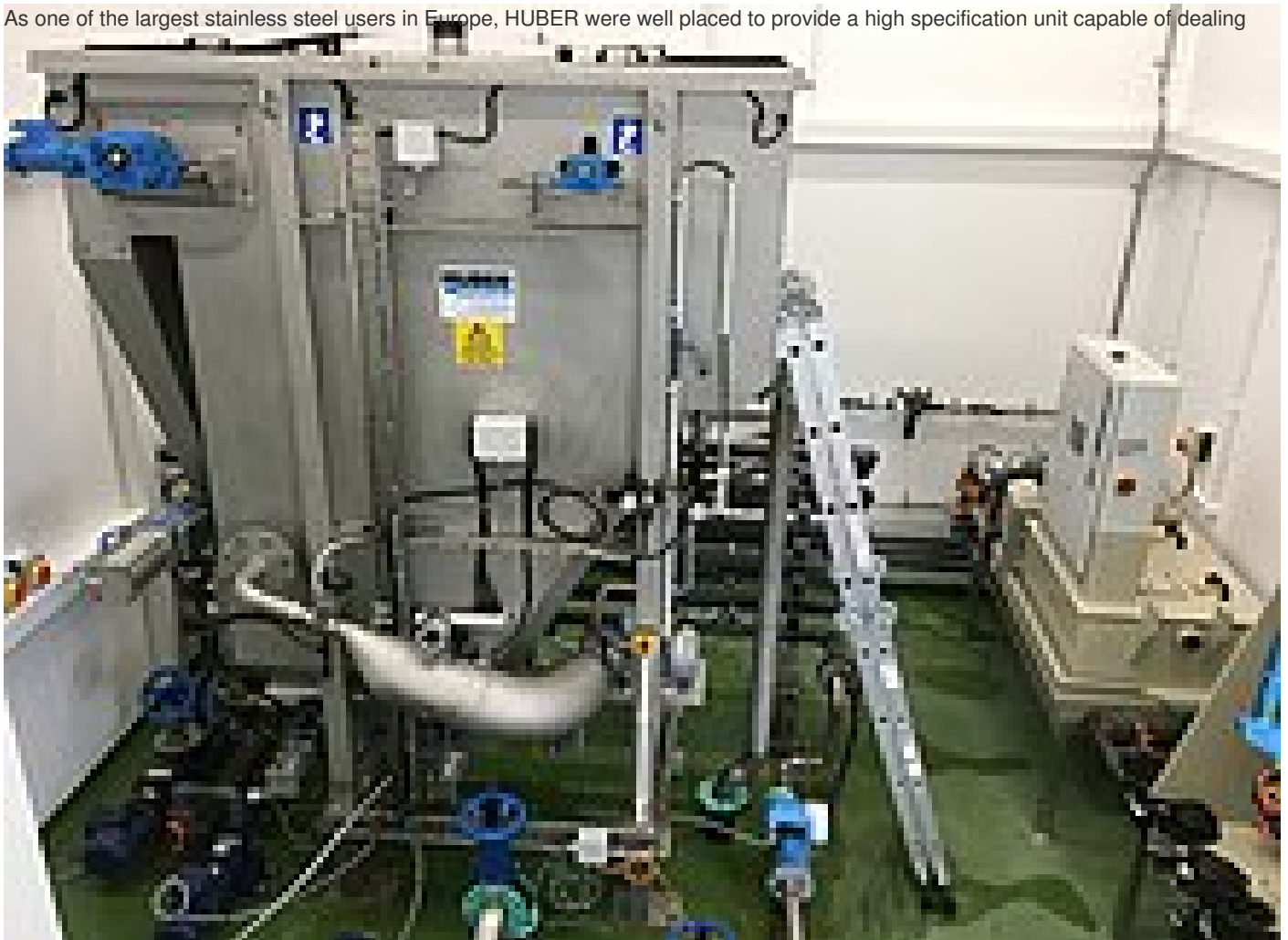
New HUBER Dissolved Air Flotation Plant HDF 1
