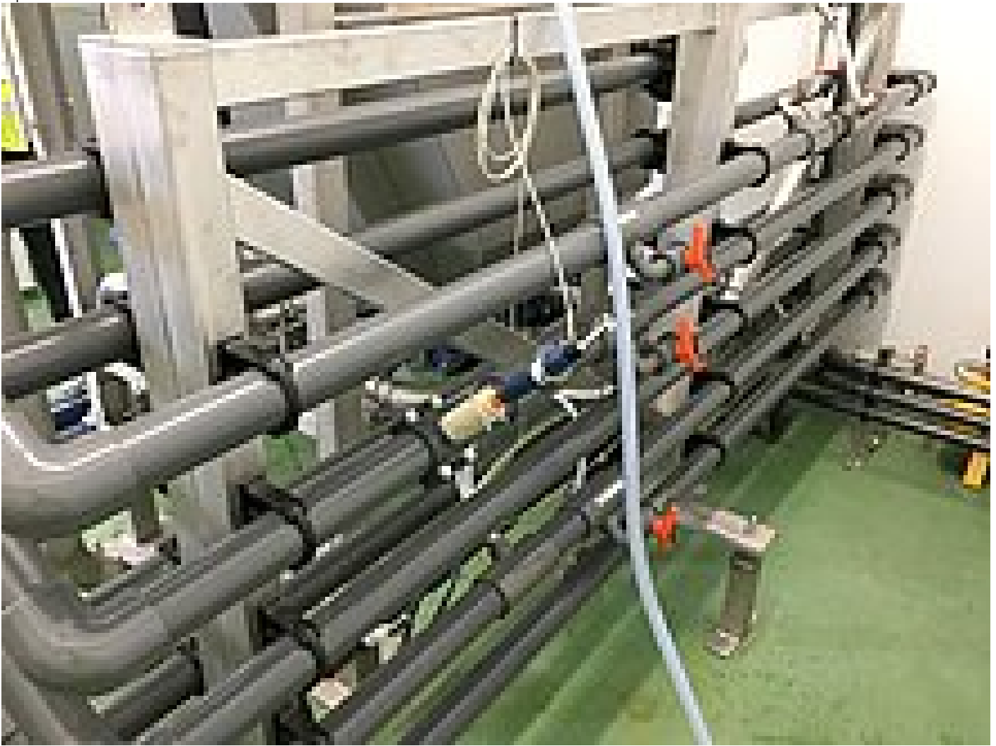
Pipe flocculator for chemical mixing
