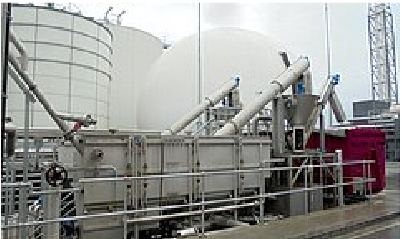
Figure 1 – Twin HUBER grit traps and grit washers
