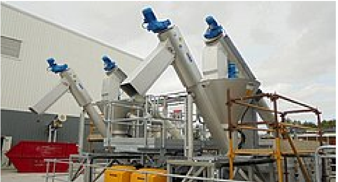
Figure 4 – Grit washers discharge over the bunded area into a skip (not shown)
