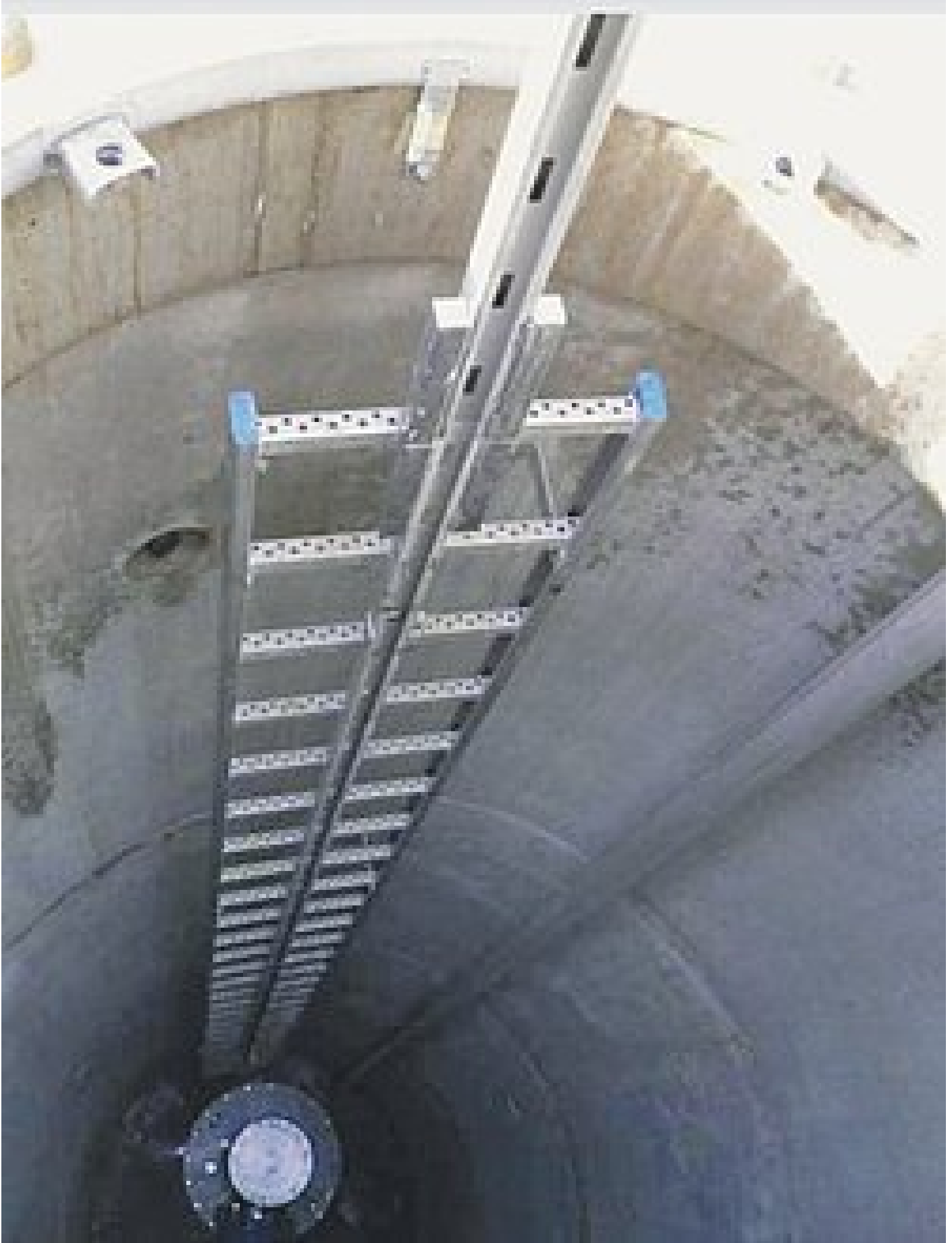
Safe access: ladder with safety guard rail
