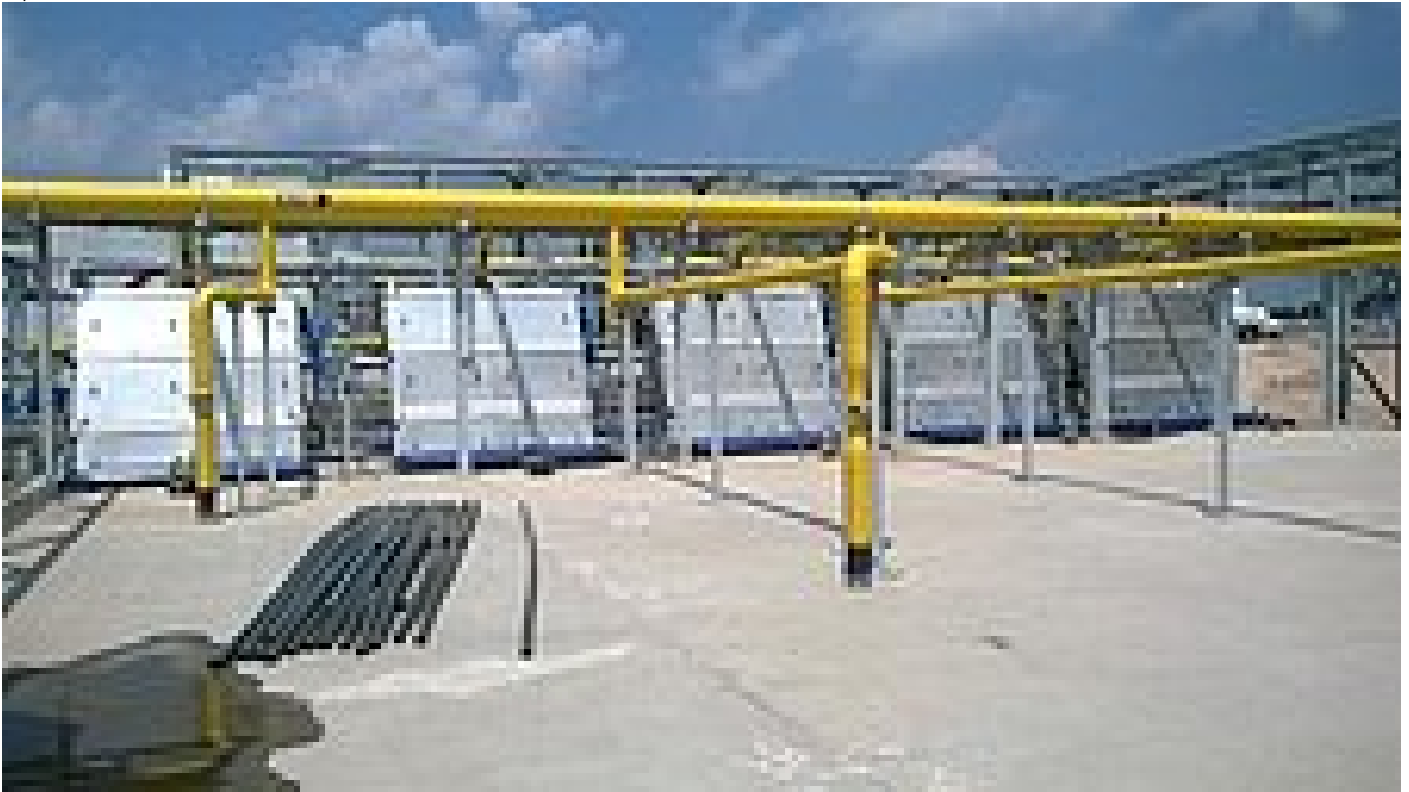
WWTP Atotonilco, the first of two coarse screen lines with 5 big HUBER RakeMax® screens, with direct discharge into a HUBER Launder Channel HLC with a length of 30m
