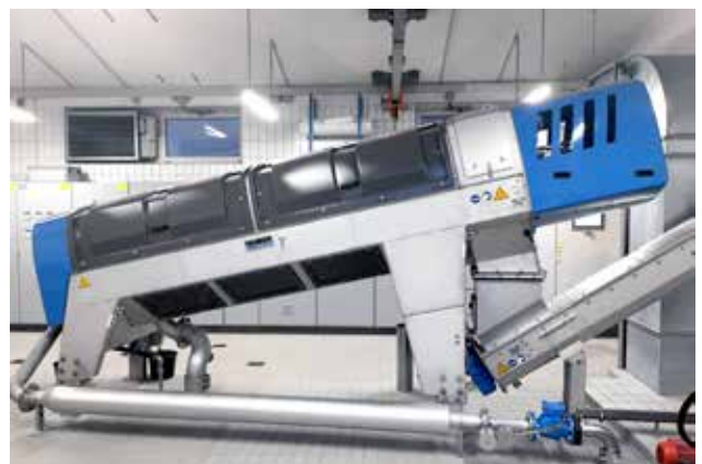
Digested sludge dewatering up to 30% DR.
