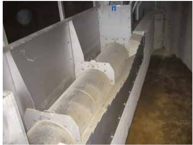
HUBER Storm Screen ROTAMAT® RoK2 with an integrated gauging weir for overflow measurement.
