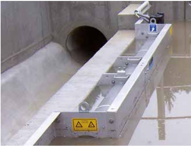
HUBER Storm Screen ROTAMAT® RoK2 before overflow.
