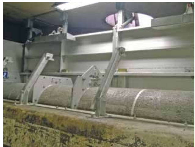
View of the upstream side and lateral screenings discharge opening.
