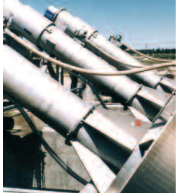
ROTAMAT® Fine screens in Argentina for the removal of solids from a sea outfall
