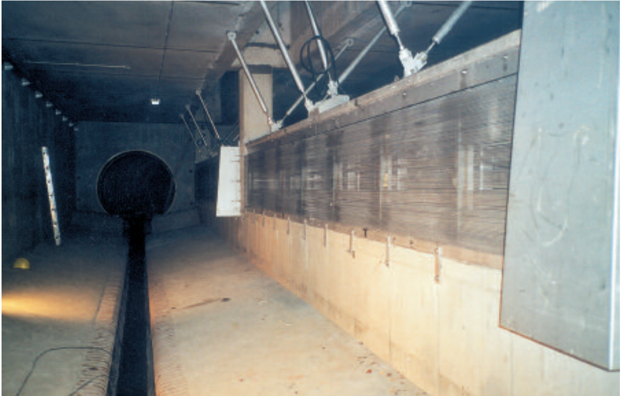
HUBER Stormwater Bar Screen HSW installed on the sill of the structure
