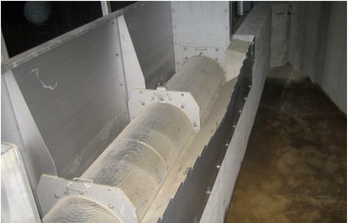
Stormwater screening combined with overflow measurement
