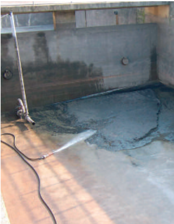
Insufficient cleaning of stormwater storage tanks after the tank emptying phase
