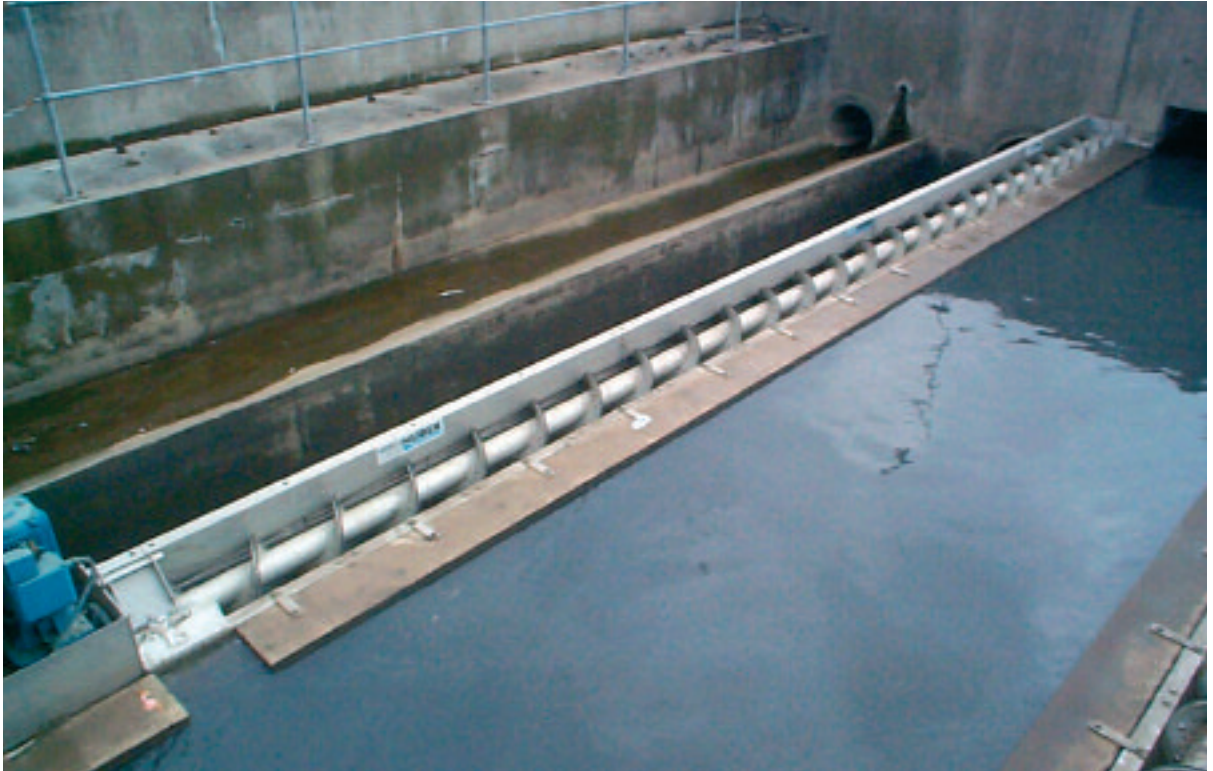
ROTAMAT® Storm Screen RoK 1 installed behind the overflow sill
