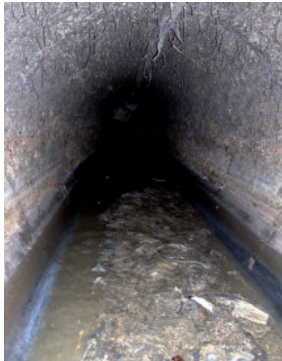
Excessive sedimentation in sewers
