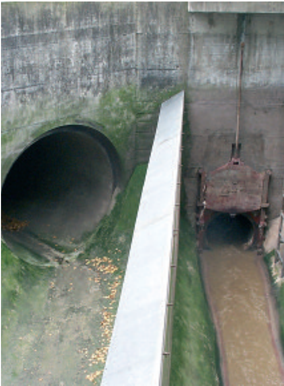
Sewers without equipment for discharge volume measurement
