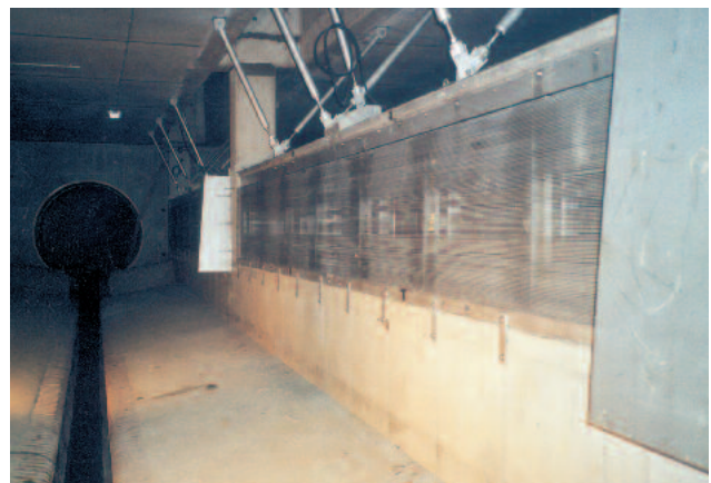
Two screens combined for an increased discharge capacity
