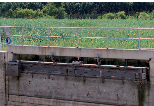
HUBER Storm Water Bar Screen HSW installed at the inlet to a soil filter
