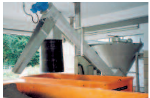
A classifying screw transports the grit from the separation room into a skip.
