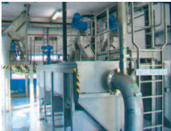
Above ground installation of an Ro 6 Grit Trap
