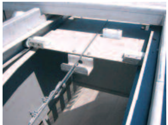
Forced grease removal by means of a paddle system
