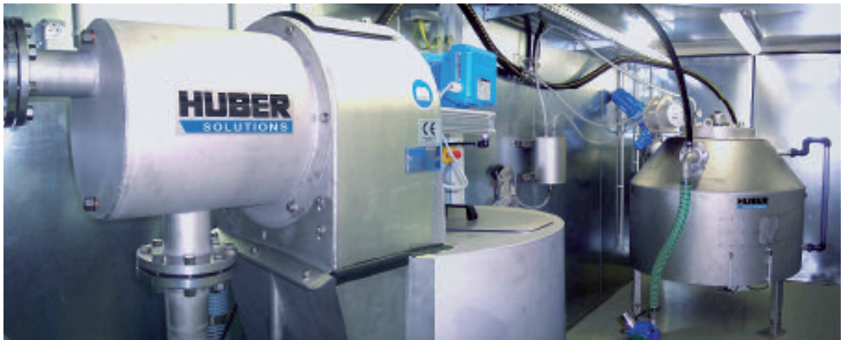
Pipestrainer used for brown water screening for later humus recovery
