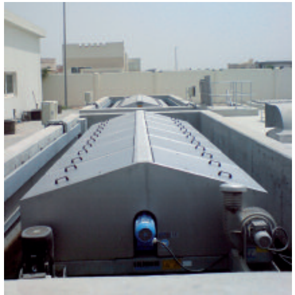
RoDisc® Rotary Mesh Screen with 20 discs installed in a concrete tank
