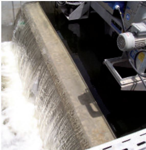
Secondary clarifier outlet with an increased solids overflow
