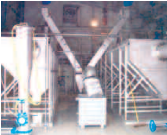
Redundant Ro 5 Complete Plants with additional Screenings Wash Press WAP
