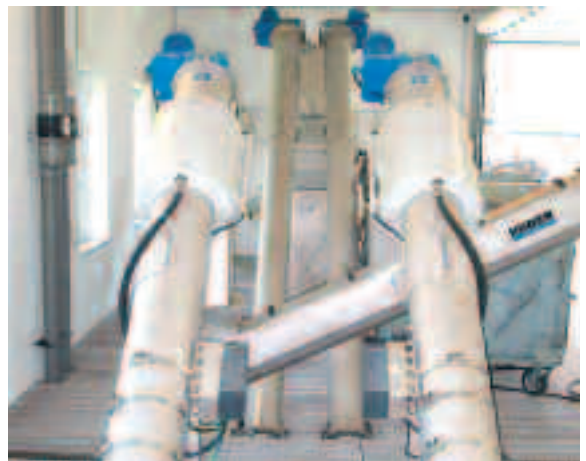
Underground, redundant Complete Plant Ro 5
