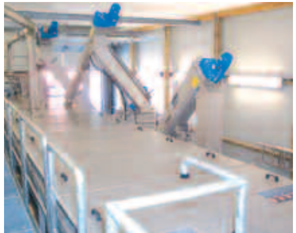
Odor-encased screenings discharge
