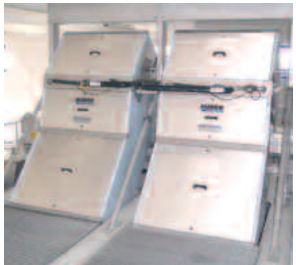
Parallel installation of two SSF screens
