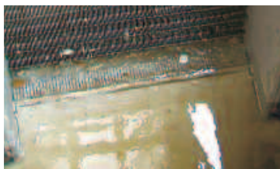
Example of a STEP SCREEN® Vertical installed such that screenings are lifted at bottom level
