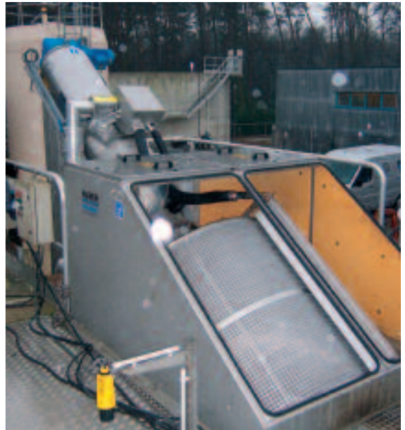
Outdoor installation of a Membrane Screen for removal of hairs and fibres prior to a hollow fibre membrane plant
