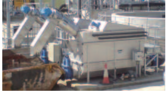
Screening of wastewater from a laundry
